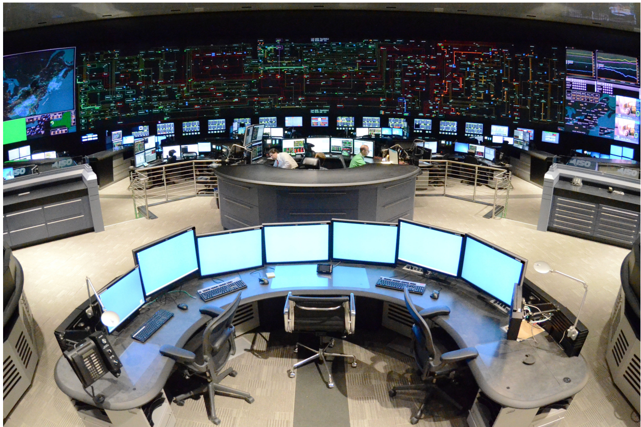
Figure 1: A large video wall display at the NYISO control center
